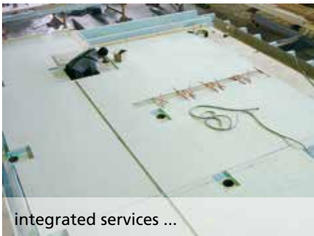
passive house roof with radiation heating ...
